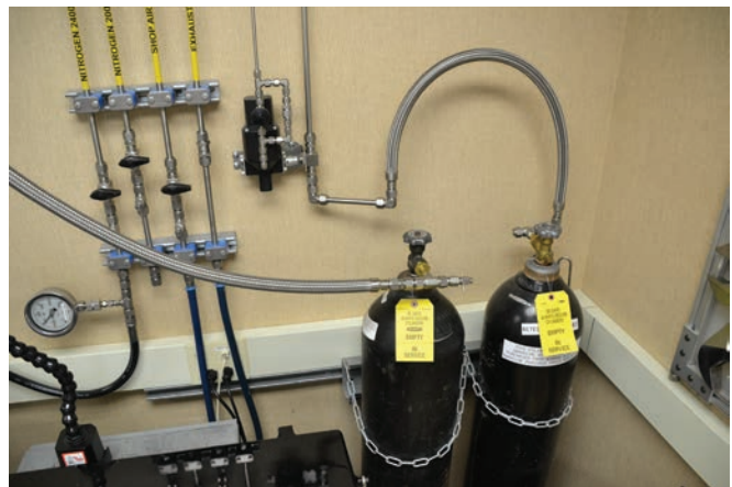
High-pressure gas distribution
